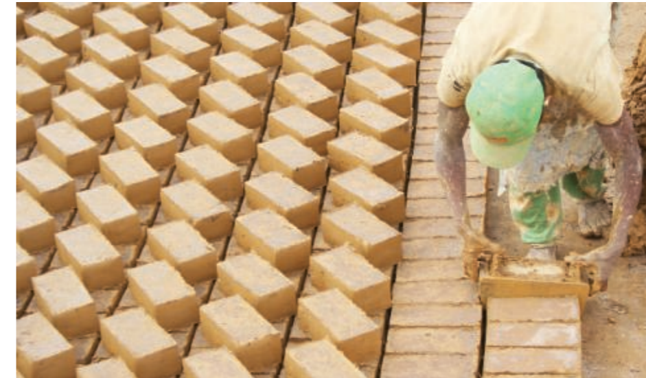
A worker forms traditional craftsmanship adobe bricks and sets them to dry in a construction site in Madagascar @ UN-Habitat
