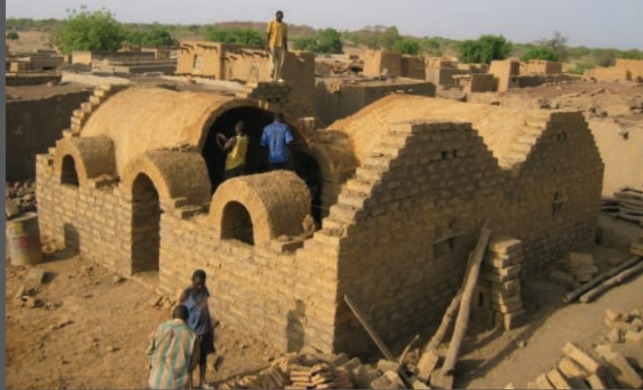
A vaulted house being constructed in Burkina Faso. Earth bricks make the structure, which is then finished with water repellent mud mortar. © AVN
